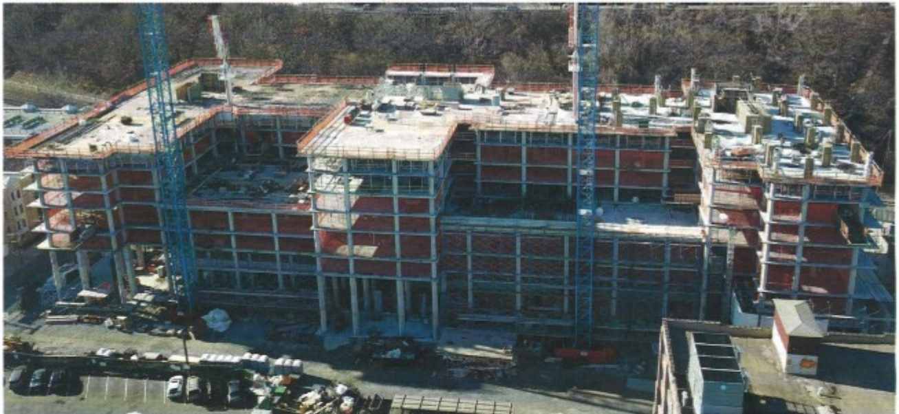
Slated to open in 2019, 700 Jackson St. is now under construction and will rise 14 stories along the Palisades of western Hoboken.
